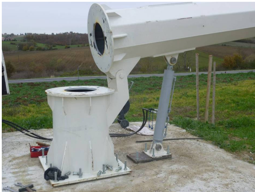
Figure 3: Lowering automated system for nacelle maintenance
